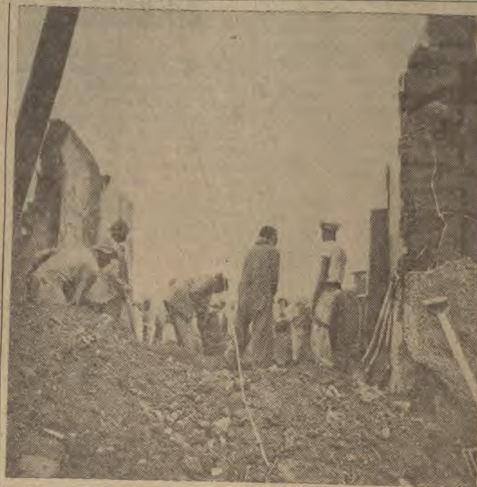
TOP: A striking view of the Albertynville wreckage, showing the first row of houses completely demolished while the others stand practically unharmed. BOTTOM: Workers shovelling away the rubble between the walls of a devastated home.
