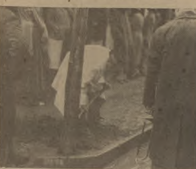
As soon as families had moved demolition squads were busy. Here electric cables are being cut as the houses are vacated.
