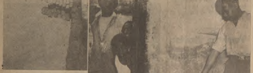
(Top) A long way from the river, this Kiptown wall was destroyed by the floods.
