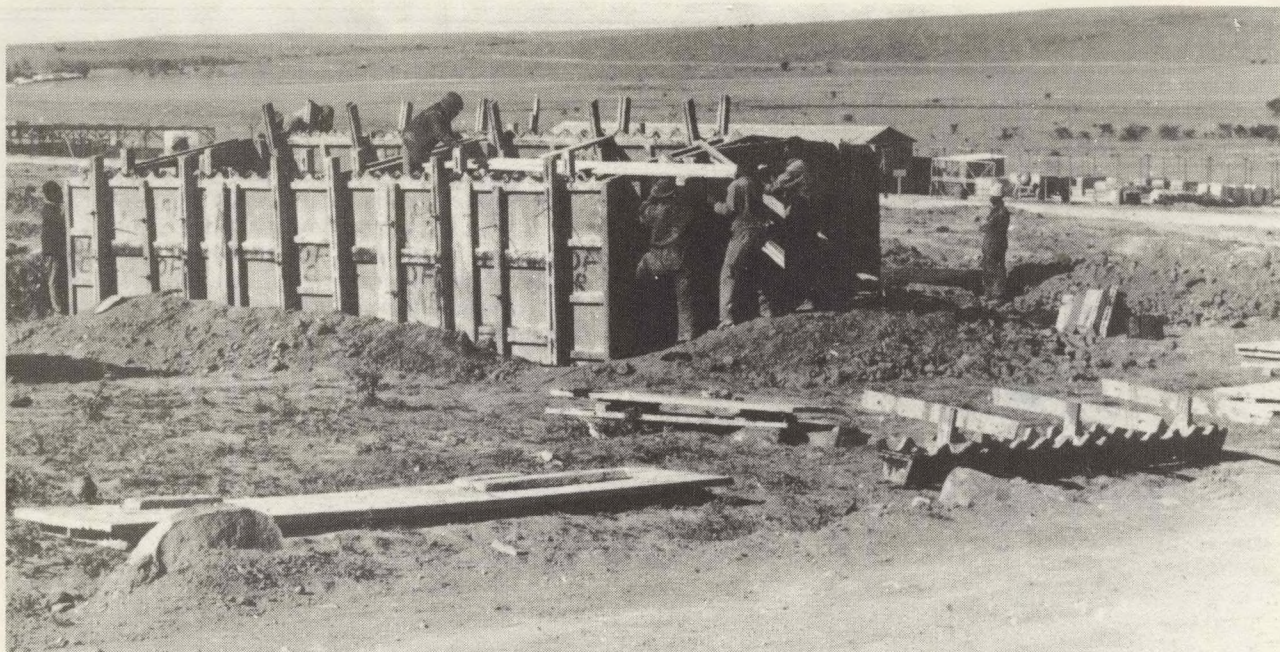
Casual labourers for the Government Department of Works, building new houses in Dimbaza. Men get £10 per month, women (widows), £3 per month.
