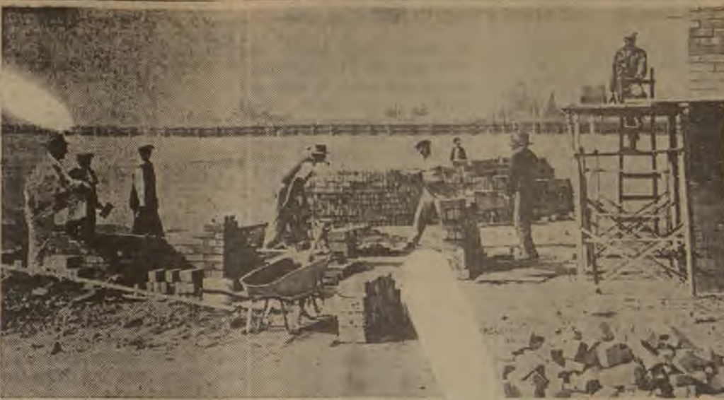
This photograph shows construction work of the Western Native Township Ground fence. This will be the first enclosed Rugby ground in Johannesburg. Officials of the Transvaal Bantu R.F. Union have always depended on donations for funds and it is hoped that this ground will greatly help them. Year after year, pleas have been made to the City Fathers in this connection and such representations made by past Committees. It is now evident, have not gone unheeded. It is understood that even new organisations are clamouring for the use of the ground.
